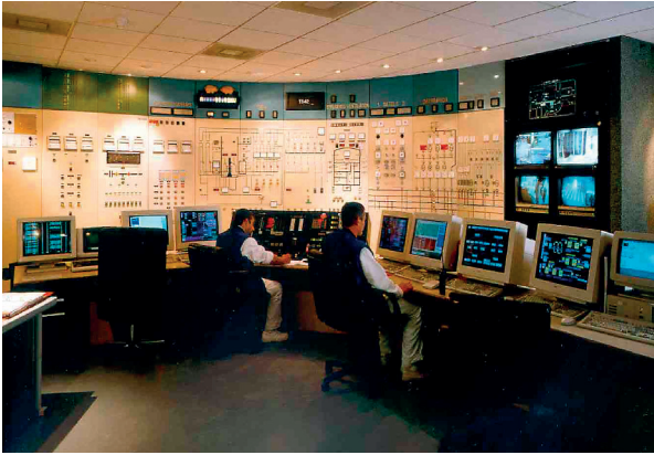
Fig. 68. OSIRIS control room.
